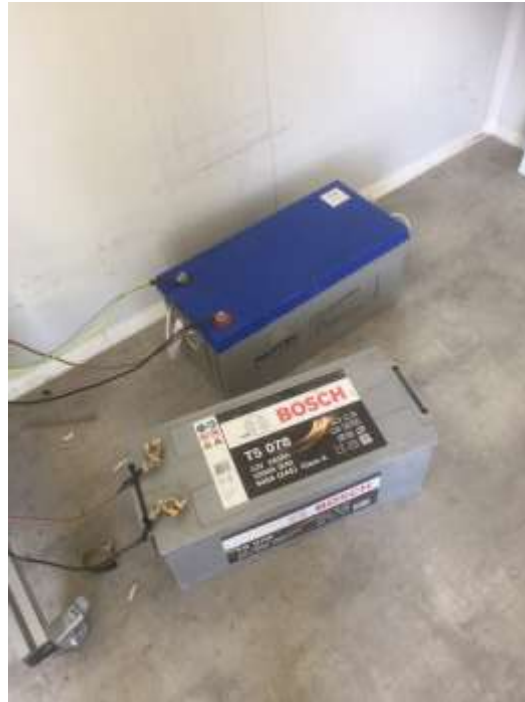
Figure_7: Batteries used for Energy Storage.
