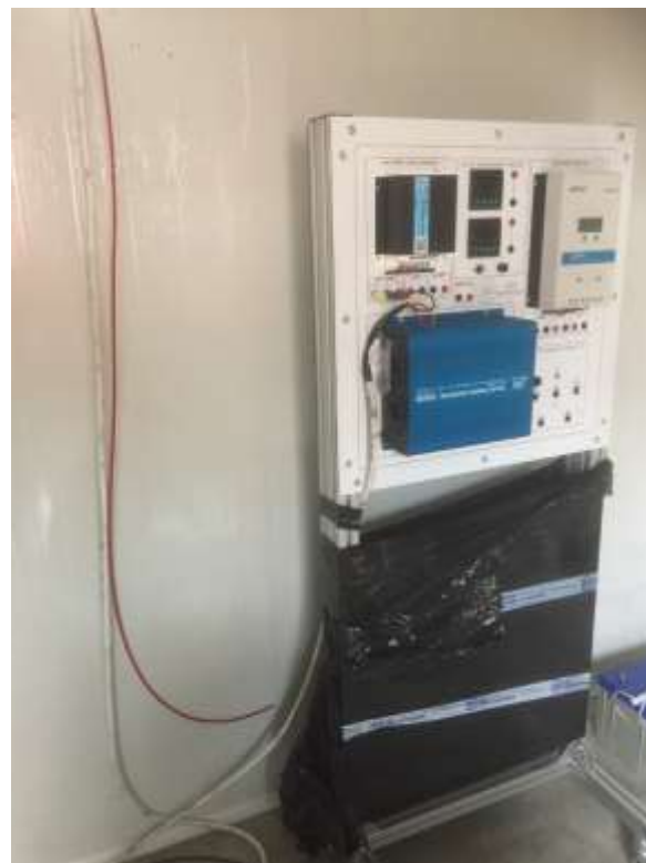
Figure_6: The complete compact control panel unit consisting of Solar Charge Controller, Wind Turbine Charge Controller, AC/DC Measurement Module, PC Interface Module, DC/AC Inverter.
