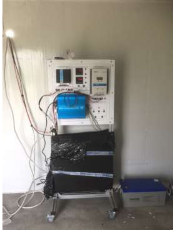
Figure_3: The complete compact control panel unit consisting of Solar Charge Controller, Wind Turbine Charge Controller, AC/DC Measurement Module, PC Interface Module, DC/AC Inverter.
