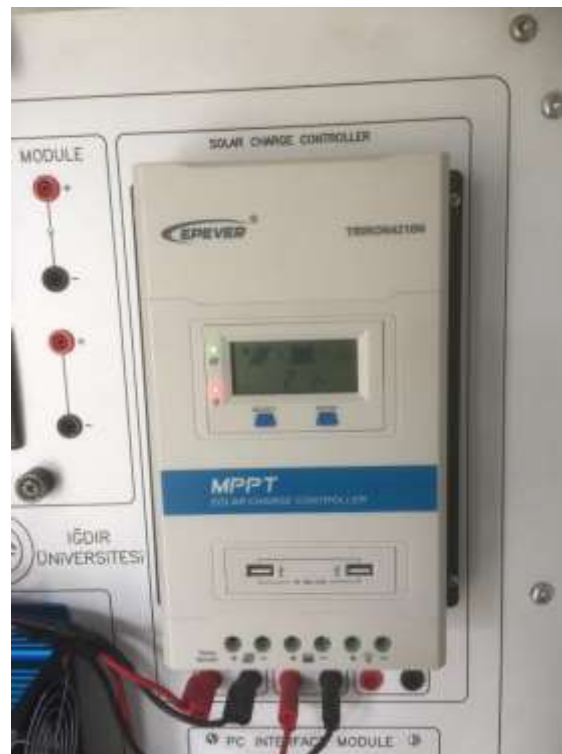
Figure_10: Solar Charge Controller.
