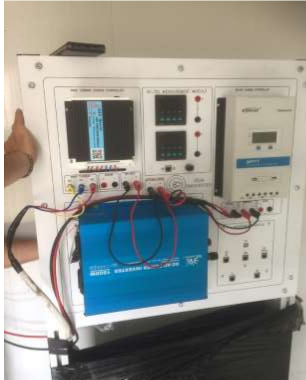
Figure_5: The complete compact control panel unit consisting of Solar Charge Controller, Wind Turbine Charge Controller, AC/DC Measurement Module, PC Interface Module, DC/AC Inverter.
